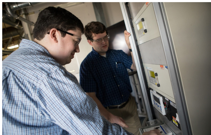
Figure 2. Researchers inspecting instrumentation measuring the outlet gas composition of the single fluid bed reactor.
