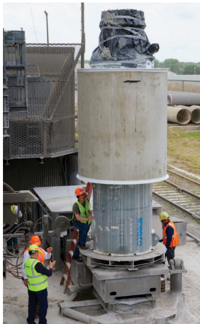
H 2 storage tank.
