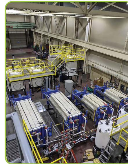
UND Coal and Mineral-Rich Tailings Filter Presses, with the Liquid Processing Tanks Featured in the Background
