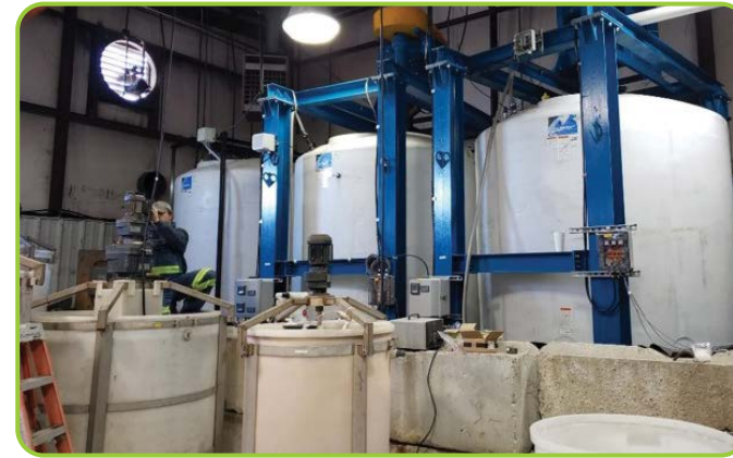
Sulfuric Acid Bioreactors
