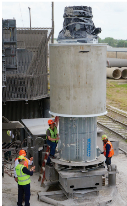
H 2 storage tank.
