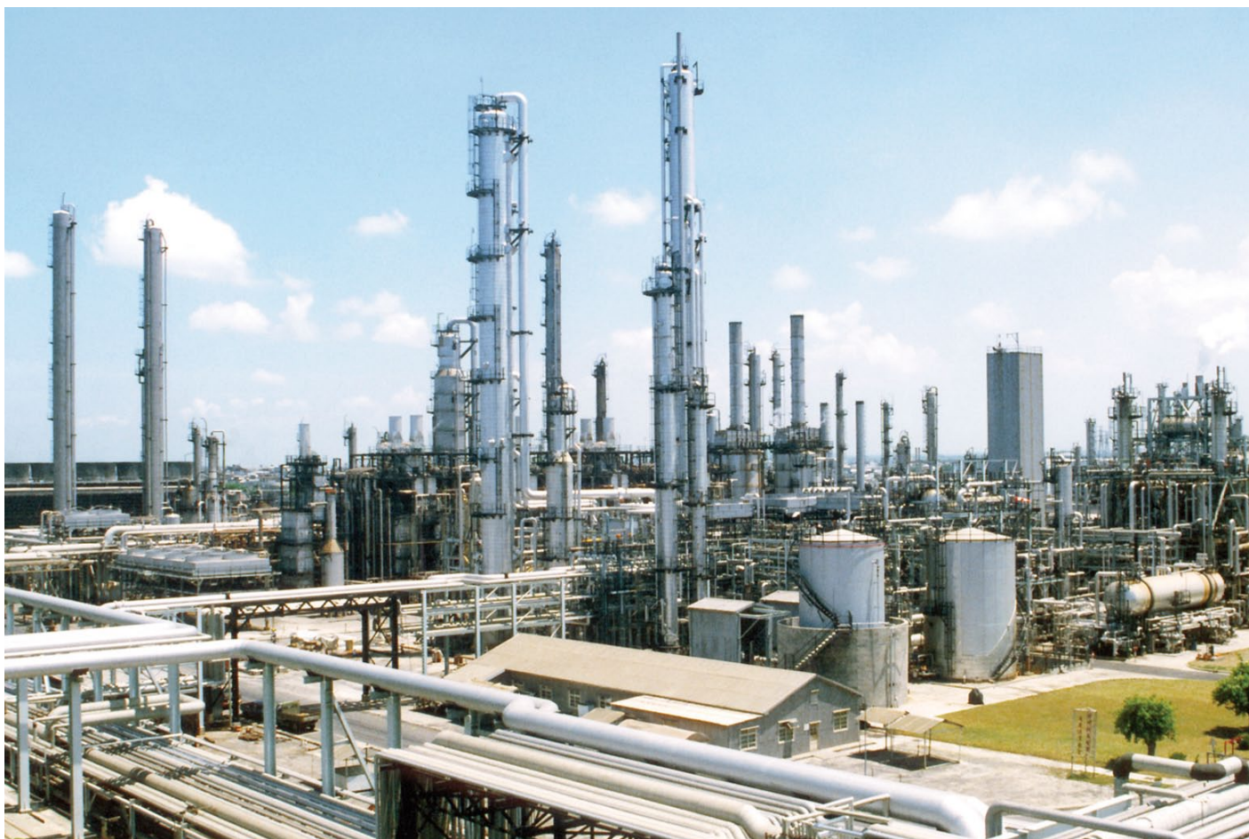
Gasification complex in Taiwan
