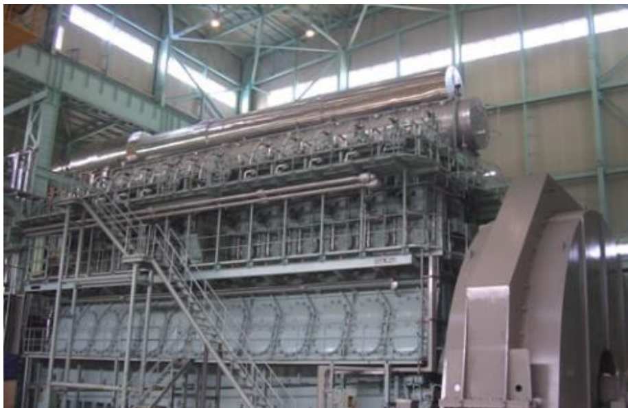
Figure 3-1 Low Speed Engine with Generator by MAN (55 MW, 120 rpm)
