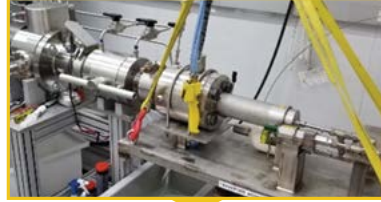
Transport Storage Chamber
