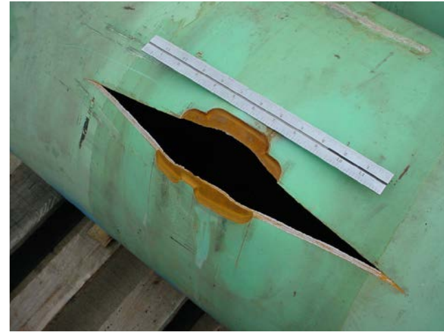
Pipe w/un-repaired damage
