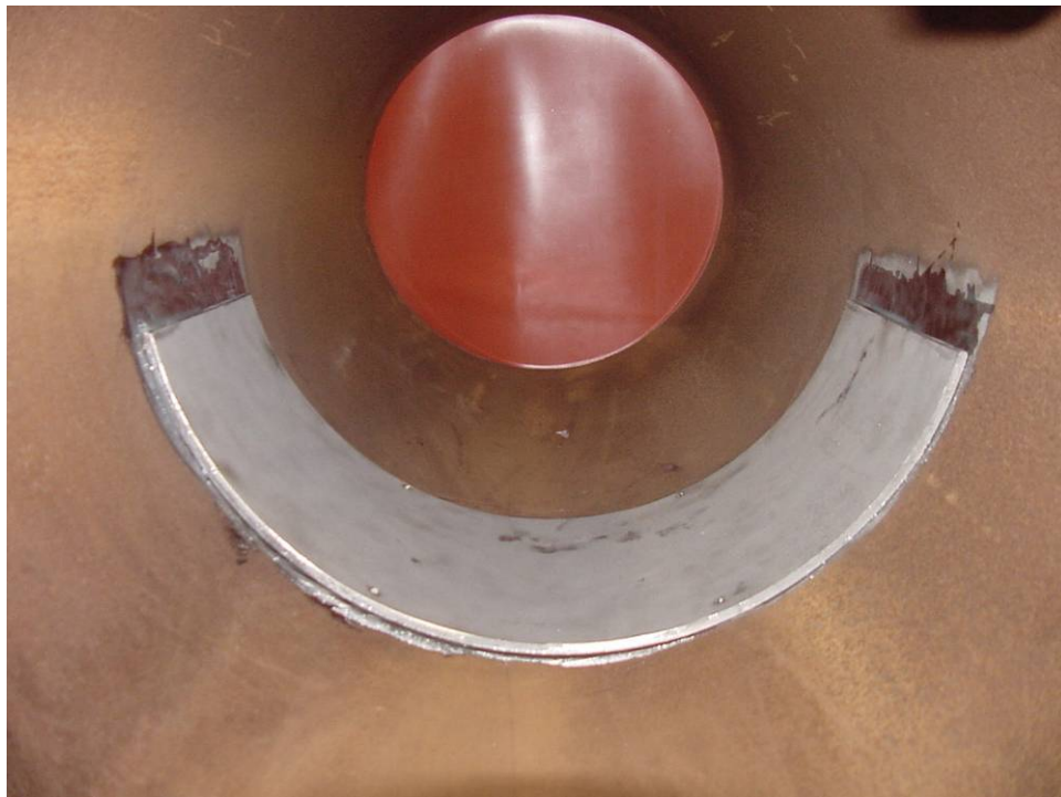
Figure 57 - Test 08 Steel Patch Prior to Epoxy Curing
