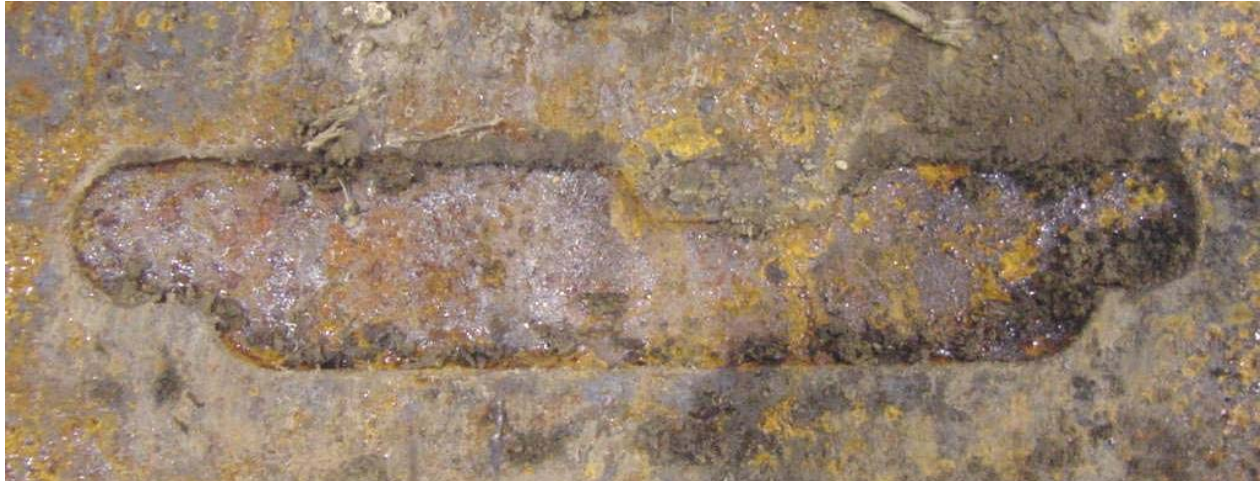
Figure 126 - Simulated Corrosion on Outside of Pipe After Weld Repair Test 01
