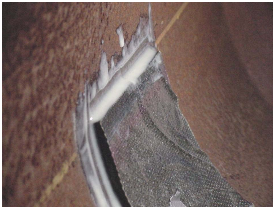
Figure 46 - Adhesive Fillet Around Test 04 CF Patch
