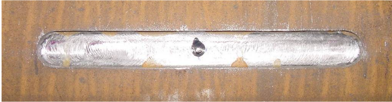
Figure 20 - Short, Extra Deep Damage with Through Hole for 609.6 mm (24 in.) Pipe
