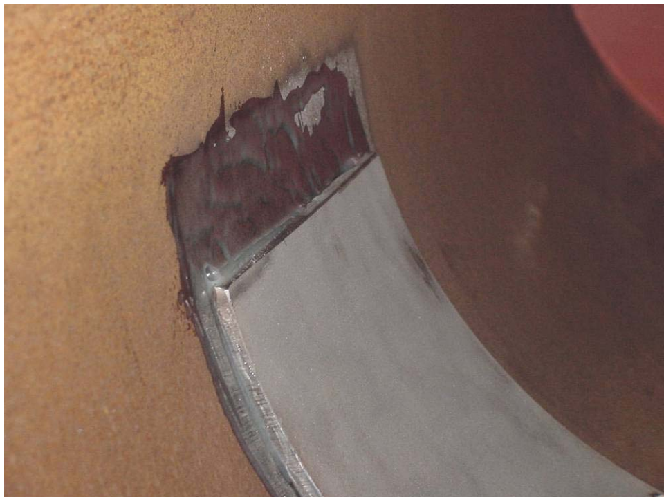
Figure 58 - Test 08 Steel Patch Prior to Epoxy Curing (Long Seam)
