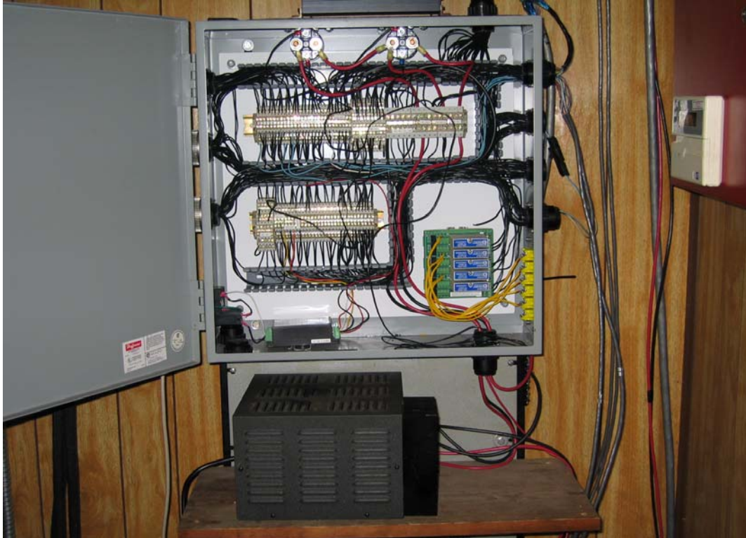
Figure 6.3. Photograph of Interior Controls Junction Box
