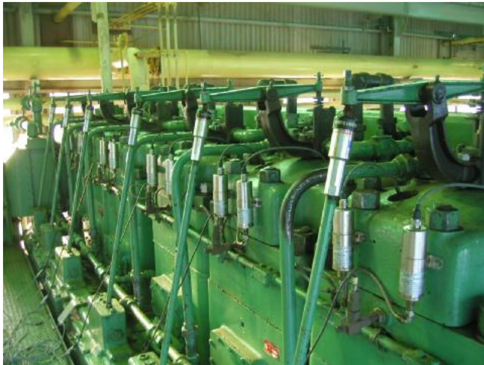
Figure 7-2. Power Cylinders; HBA-6T at El Paso Station 823; April 2004
