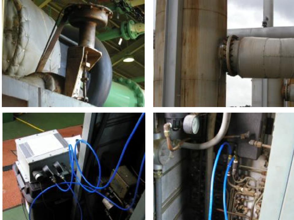
Figure 7-7. Element of Wastegate Control for Equivalence Ratio; HBA-6T at El Paso's Station 823; April 2004
