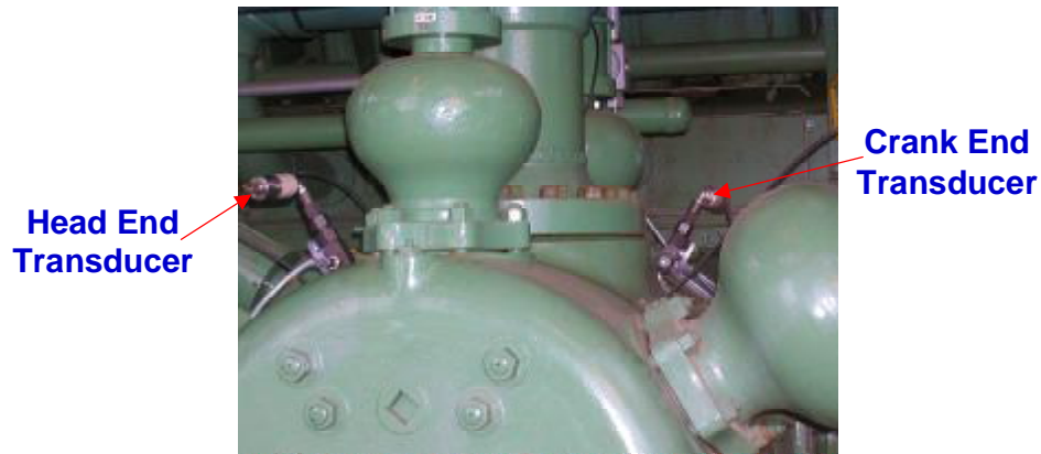
Figure 3-3. Compressor Cylinder and Pressure Transducers on each End (Williams Station 40; August 2003)
