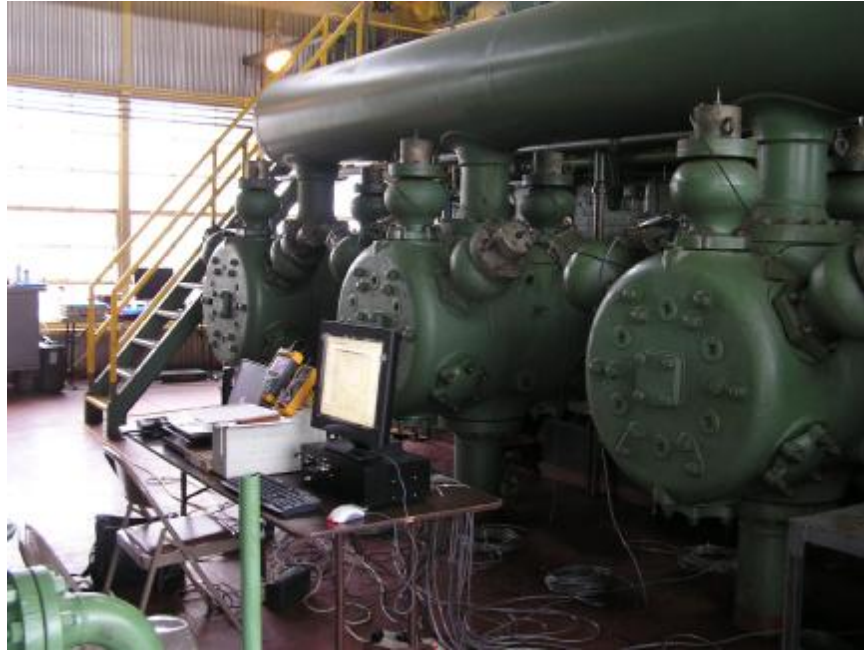
Figure 6-1. GMW10 Compressor Cylinders with Pressure Transducer Installed (Williams Station 60; February 2004)
