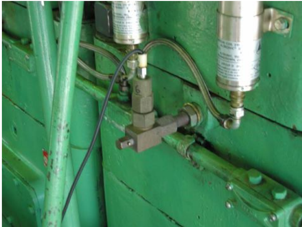
Figure 7-5. Power Cylinder Pressure Transducer; HBA-6T at El Paso's Station 823; April 2004
