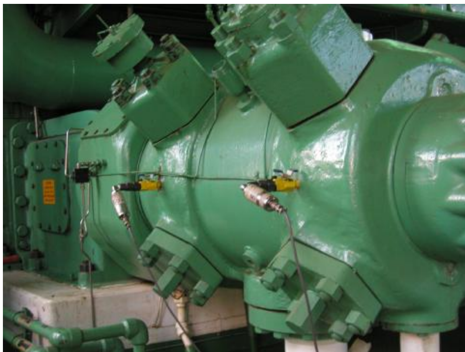
Figure 7-4. Compressor Cylinder with Pressure Transducers Installed on Head and Crank Ends; HBA-6T at El Paso's Station 823; April 2004
