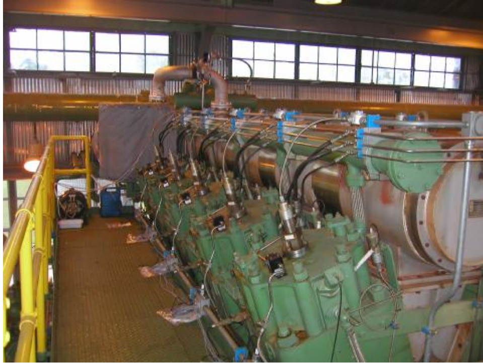
Figure 5-2. Power Cylinder, Left Bank; (Williams Station 40 (Sour Lake); August 2004)
