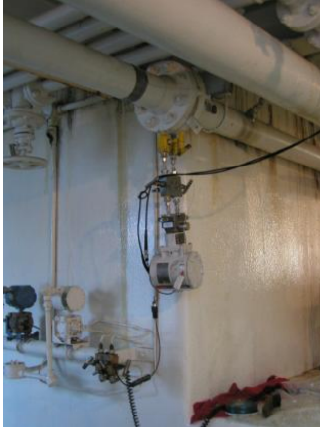
Figure 3-17. Fuel Flow Measurement using Emerson Flobas 103 Transmitter (HBA-6T; El Paso Kinder Station; April 2004)
