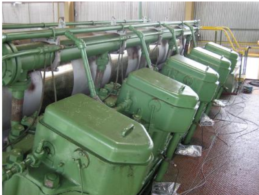
Figure 6-2. GMW10 Power Cylinder with Pressure Transducers Installed (Williams Station 60; February 2004)
