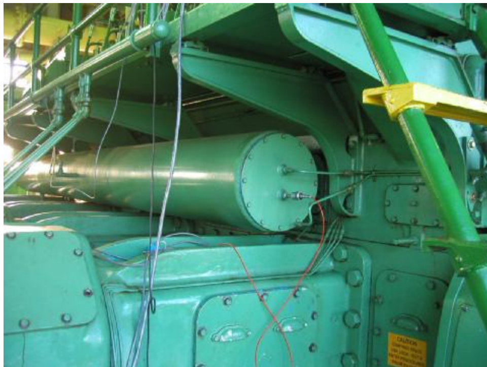
Figure 7-6. Air Manifold Pressure Transducer; HBA-6T at El Paso's Station 823; April 2004
