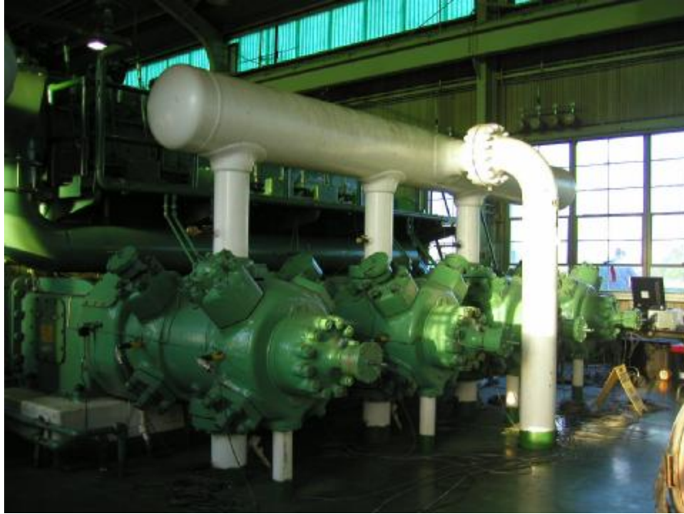
Figure 7-1. Compressor Cylinders; HBA-6T at El Paso Station 823; April 2004
