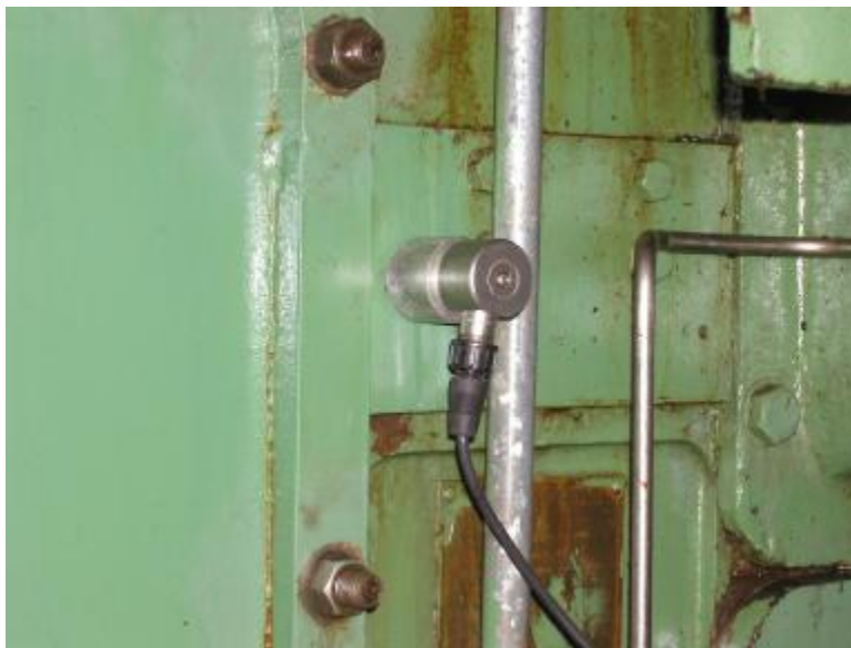
Figure 3-10. Accelerometer Mounted on Frame (GMW10; Williams Sour Lake Station; August 2003)
