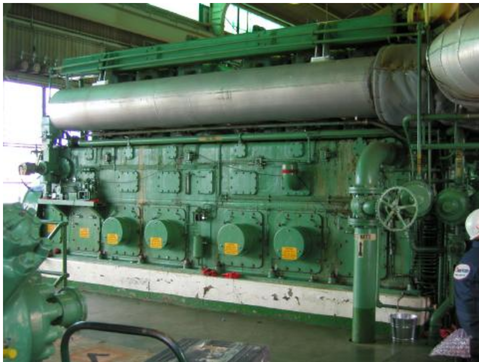
Figure 7-3. Back View of Engine; HBA-6T at El Paso's Station 823; April 2004
