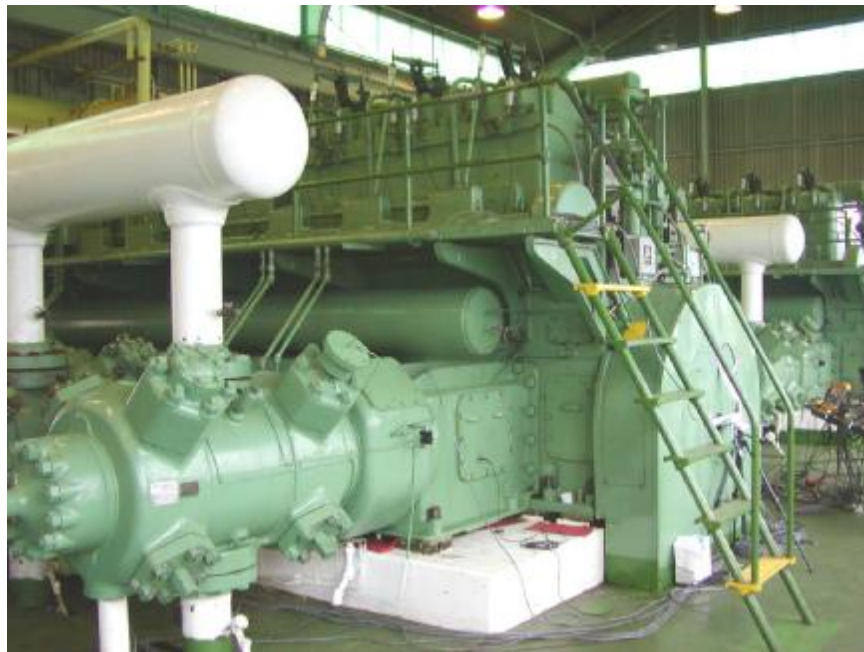
Figure 3-5. Initial Site Test (HBA-6T; TGP Kinder Station; April 2003)
