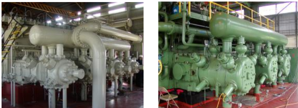
Figure 1-1. TLA6 (2000 HP) and GMW10 (2500 HP) in Pipeline Service
