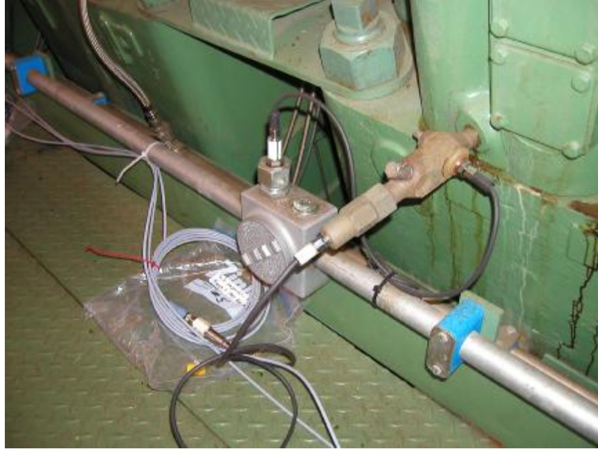
Figure 3-4. Details of Power Cylinder Pressure Transducer Installation (Williams Station 40; August 2003)
