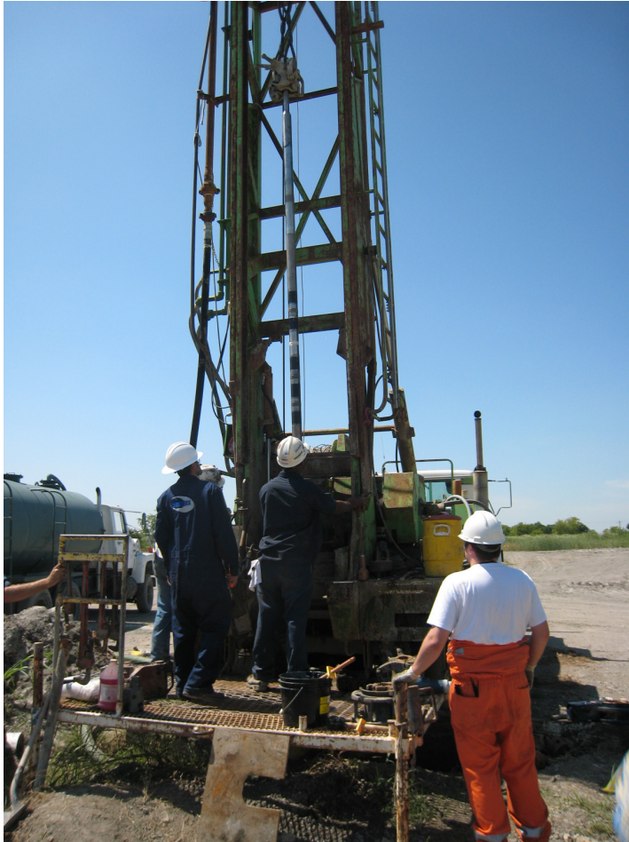
Making up BHA – 1 st Day of Test. Resistivity Collar Hanging in Derrick.
