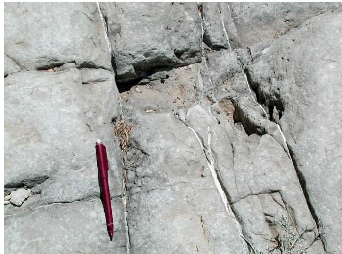
Figure 19. Two orthogonal sets of joints near a large normal fault. The joints filled with calcite (veins) are parallel to the fault trace. The set normal to the fault trace, therefore normal to the maximum horizontal stress, is closed. Permian rocks at Algerita Escarpment.
