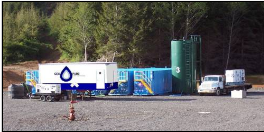
Figure 10 GeoPure Water Technologies, LLC field unit on location in Oregon
