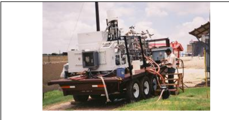
Figure 8 shows the GPRI desalination trailer at the water treatment plant on the A&M campus.
