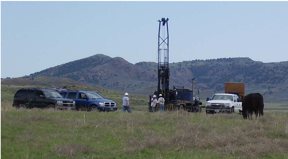
Drilling below an On-Channel CBNG Impoundment in the Prairie Dog Creek Watershed, Wyoming
