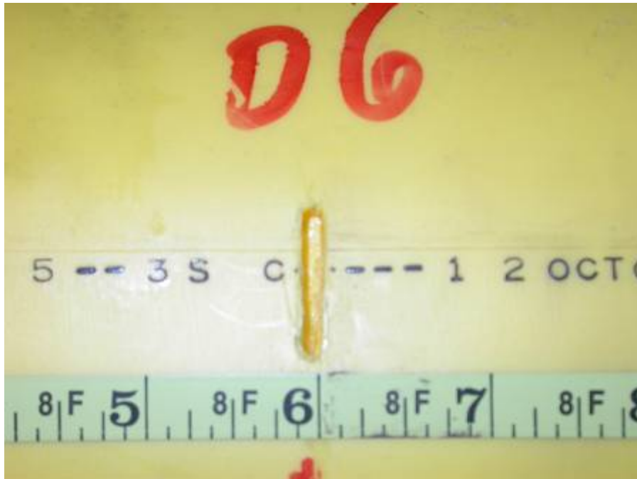
Figure 5-8. Defect D12 (D6)
