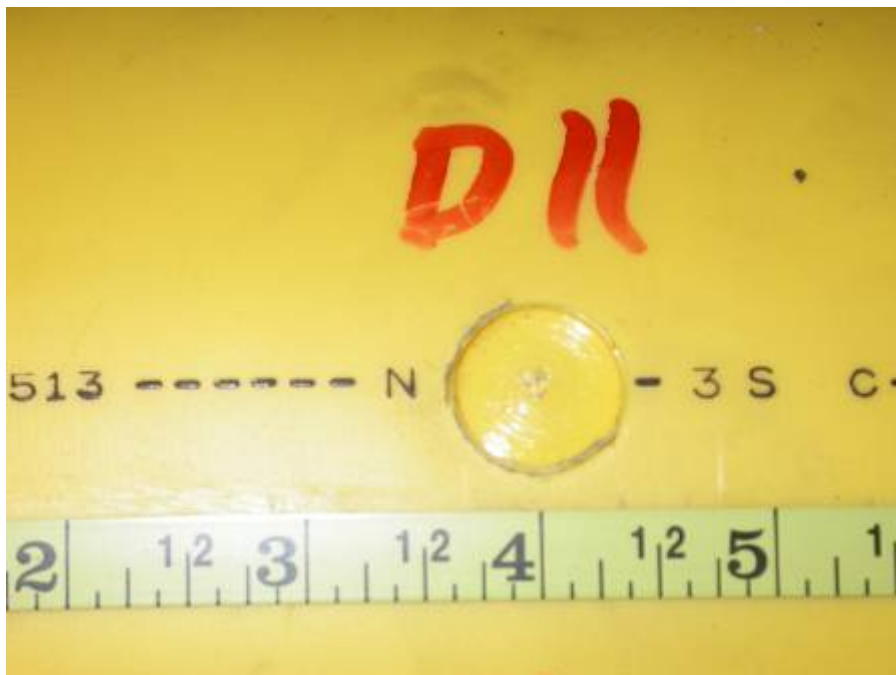
Figure 5-13. Defect D19 (D11)
