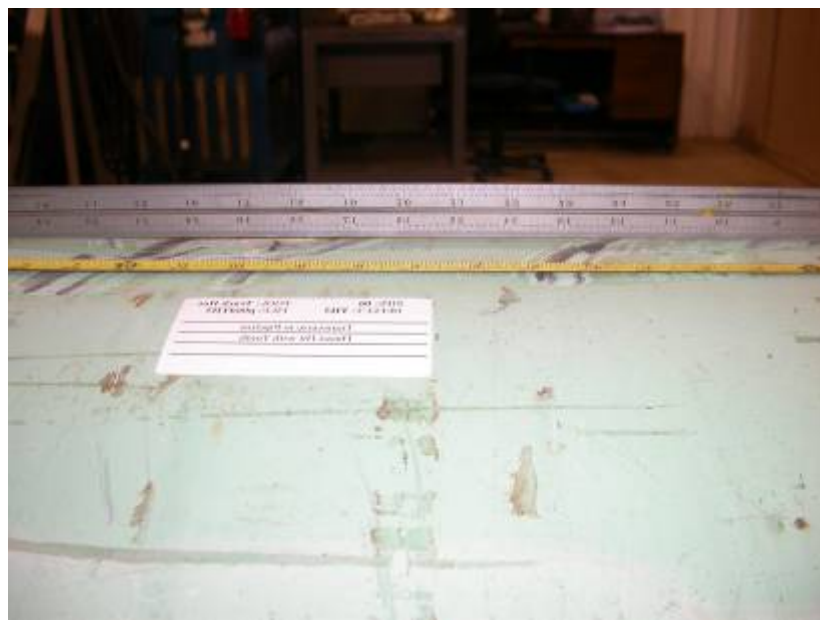
Figure 3-10. Defects D4 and D5 (p06dTH3)
