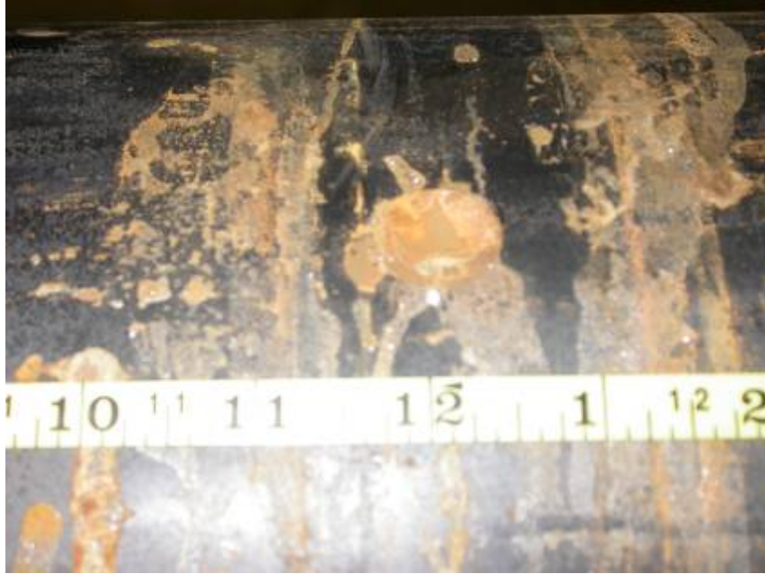
Figure 2-37. Defect P3-14 (Defect 9)
