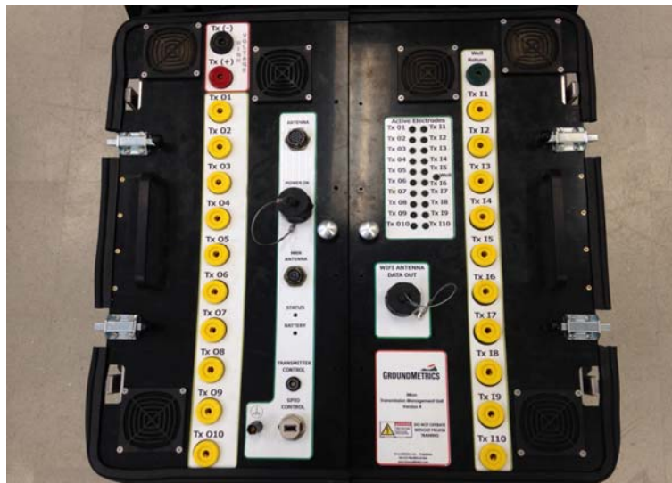
Figure 1. Current monitoring system
