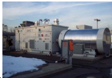
Outdoor Pads for 400 kW Grid Connected System Tests
