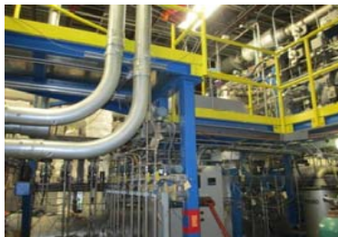
Facilities for up to 400 kW Stack Tests
