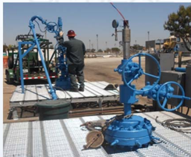
Downhole CO 2 monitoring
