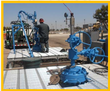
Downhole CO 2 monitoring
