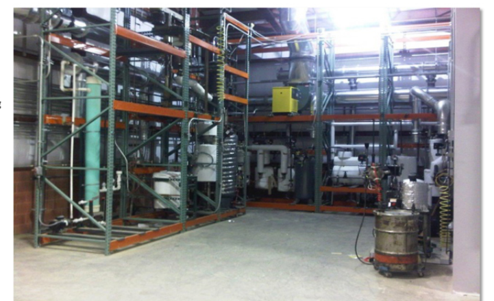
Quantex 1 TPD Continuous Coal Liquefaction System
