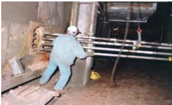
Fireside corrosion during in-plant testing with high-sulfur coal.
