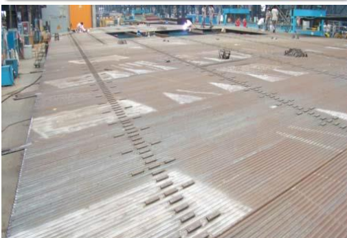
Boiler wall layout in shop.
